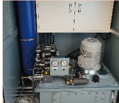
Hydraulic Power System for MLA
